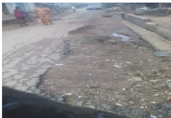
Figure 5. Deplorable condition of Isolo and Ijomu interchange owing to poor maintenance. Source: Field Survey (2019)
