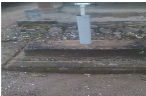
Figure 4. Non-functioning water-tap due to poor maintenance in Araromi street. Source: Field Survey (2019)
