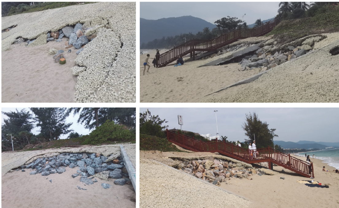
Figure 8. Series of Photos Showing Damage to the Protective Slope Project (Photographed on 2024.12.16)
