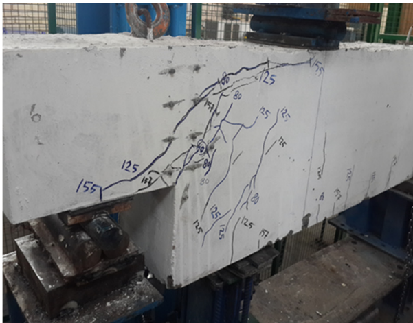
Figure 22. Cracks Modality for specimen DBNCR1.5
