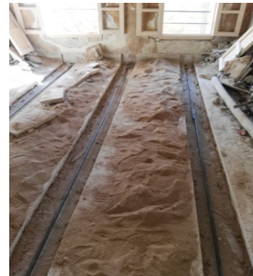
Figure 35. Pre-stressing bars buried under tiles (Hammoud J., 2019)
