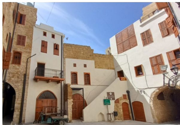
Figure 27. Applying three coats of non-hydraulic lime on the stone facade enhances the aesthetic appeal by showcasing its natural color. Each layer is meticulously applied, starting with a rough scratch coat to provide a strong foundation, followed by a smoother coat, and finishing with a finely textured top coat. This process not only ensures durability but also highlights the lime's inherent beauty, creating an elegant look on the stone surface. (Hammoud J., 2022).
