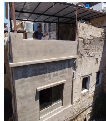
Figure 18. Addition of floor with inconsistent material in Musalkhieh street(Hammoud J., 2022)
