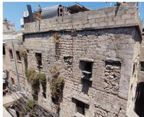
Figure 17. Deteriorated concrete string course and closed openings in the Musallabiyyeh market street
