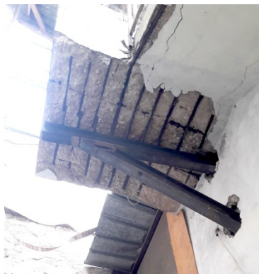
Figure 16. Balcony hazardous element in Furn el Saha square
